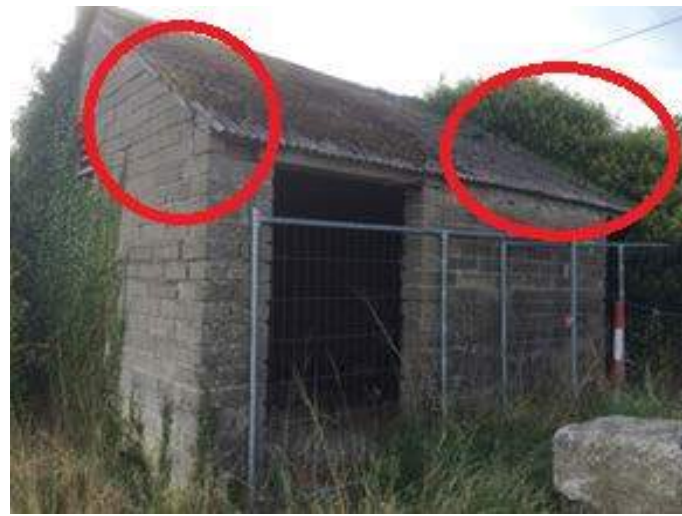
Photo 11.1: Building (shed) with cracks in brick work and dense ivy cover. Point A on Figure 12.2.
